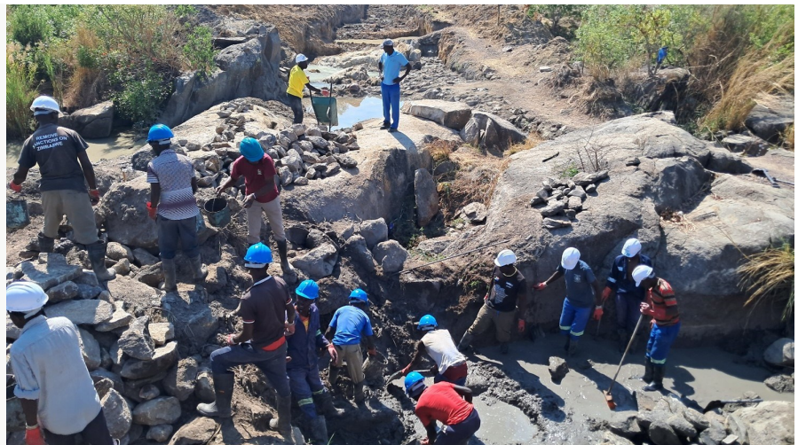
MEN AT WORK: Community volunteers working during the rehabilitation of the new dam wall. Photo for by Caritas Chinhoyi for CRS.
