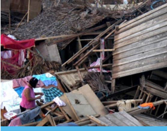
The poor are the most vulnerable to natural disaster. This photo shows the destruction to homes after a typhoon in the Philippines. Photo by Jennifer Hardy/CRS
