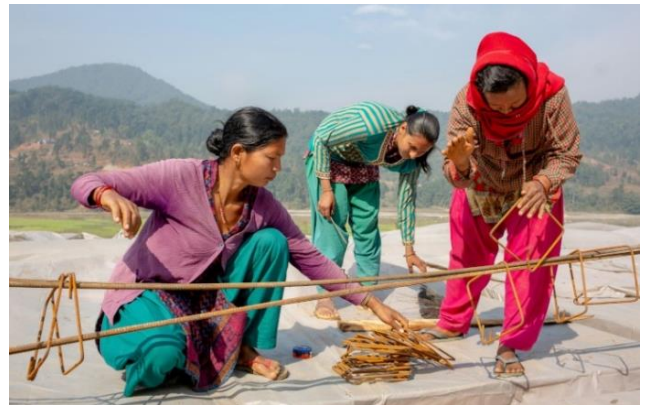
After devastating earthquakes hit Nepal in 2015, CRS trained local masons in earthquake-resilient construction techniques. Photo by Jenifer Hardy/CRS
