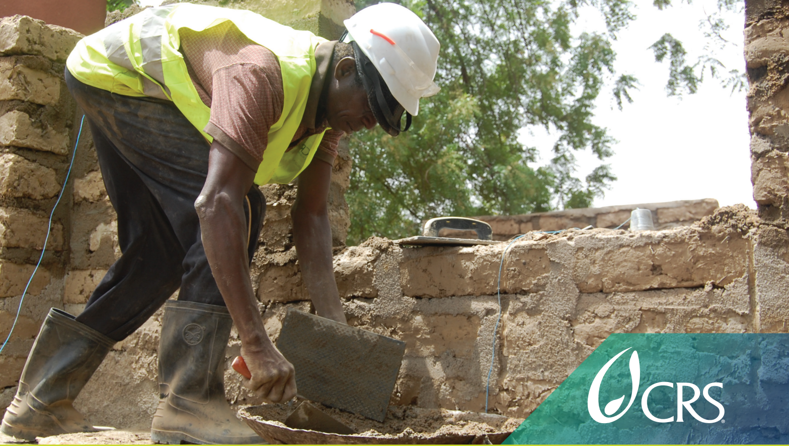
A local mason, trained by the CRS Sandji Ko project, models resilient construction practices for a flood-prone community. Photo by CRS staff
