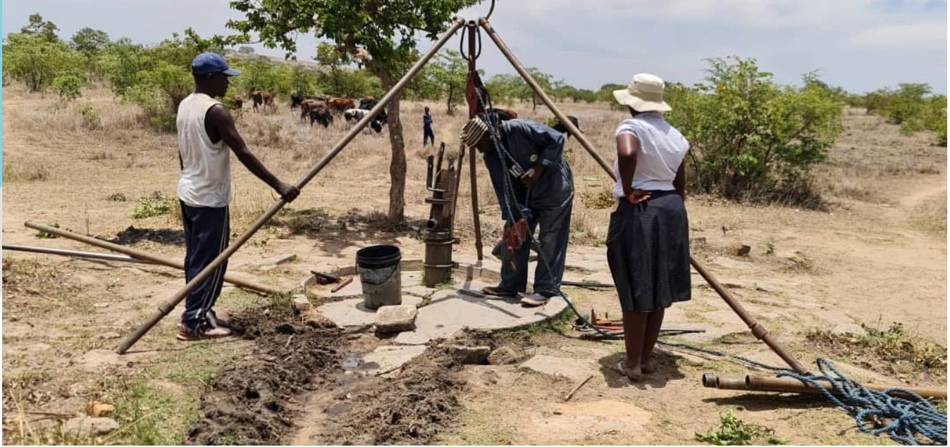
Rural Infrastructure Development Agency (RIDA) setting up for borehole rehabilitation in Buhera district. Photo by Caritas Mutare for CRS
