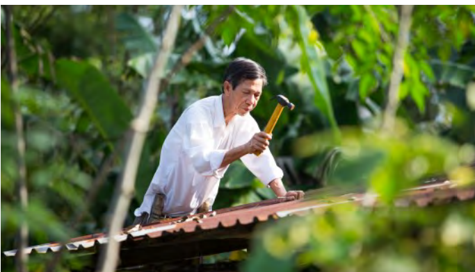
Cao Xuan Hoa adds the finishing touches to a new section of roof, damaged by Typhoon Damrey 2017.
