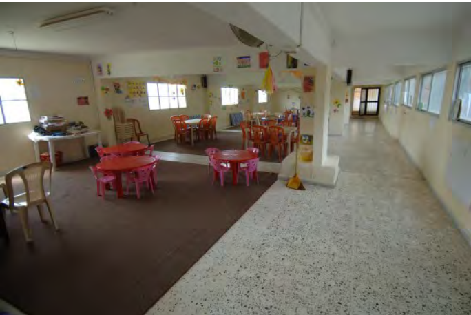
A kindergarten rehabilitated by CRS in the basement of a municipal building damaged by bombing during the war, 2007.
