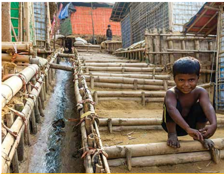
Through a CRS cash-for-work activity, Rohingya refugees used local materials to build structures such as drainage and terraces to mitigate erosion and flooding in the refugee settlement. Photo by Christopher Reichert/CRS
