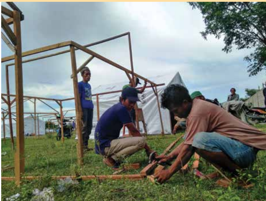
Community members construct temporary shelters for those whose homes were destroyed. Photo by Maria Josephine Wijastuti/CRS
