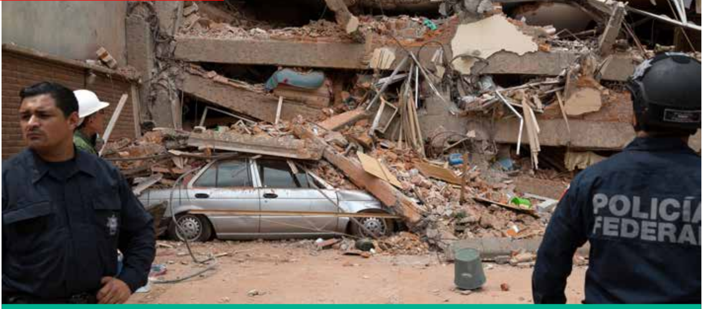
A collapsed building in the Lindavista neighborhood of Mexico City. Photo by Benedicte Desrus/Alamy Live News
