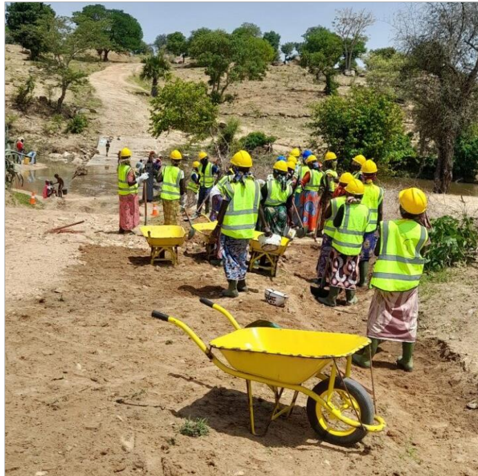
The STaR project uses a mixed approach to infrastructure improvement, employing both the private sector and men and women from participant communities via Cash-for-Work. Photo by CRS Staff.
