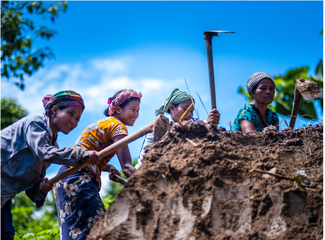
A group of cash-for-work project participants builds a new road near their village in Bangladesh. The road is connected by a bridge constructed with local materials like bamboo. Cash-for-work programming helps people earn money by working on projects that support disaster risk mitigation efforts in vulnerable communities. Photo by Amit Rudro for CRS
