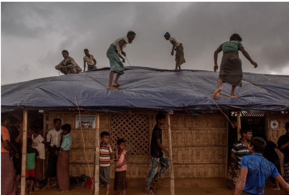
Rain-proofing a building in a Rohingya refugee camp in Bangladesh. Bangladesh hosts close to 1 million Rohingya refugees from Myanmar, and is one of the most risk-prone countries to climate disasters. [Ismail Ferdous for CRS]
