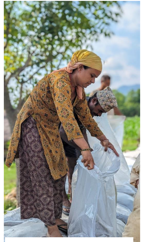
Community members constructing a sandbag embankment in the Banke district of Nepal. In October 2022, flooding in the district displaced over 1,000 people and swept away 50% of paddies. [Bibek Shrestha for CRS]
